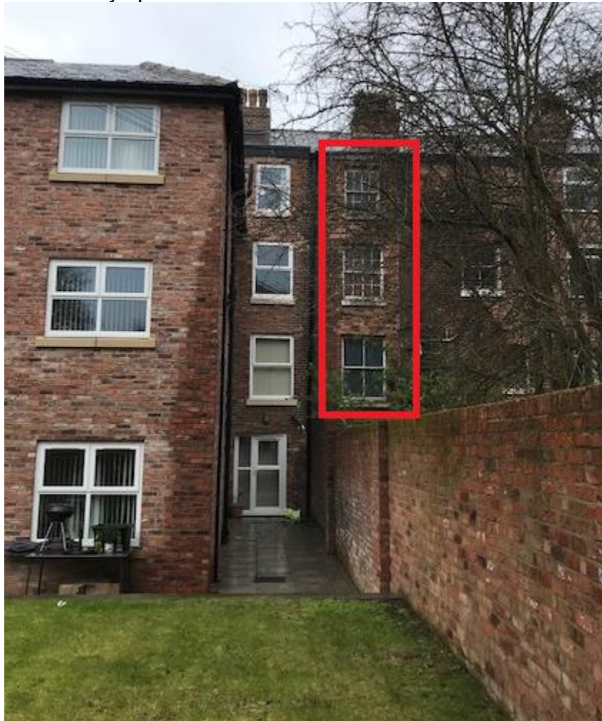
Rear of application property – the unauthorised extension is to the left - showing relationship with windows in adjoining 361 Wilmslow Road
